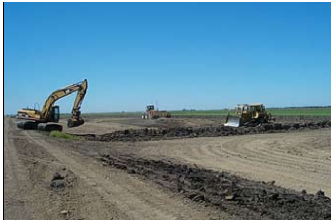
Figure 4. Restoration and Enhancement Construction. Earth work underway in the 2004 marsh construction project on the Conservancy's Cummings tract.
